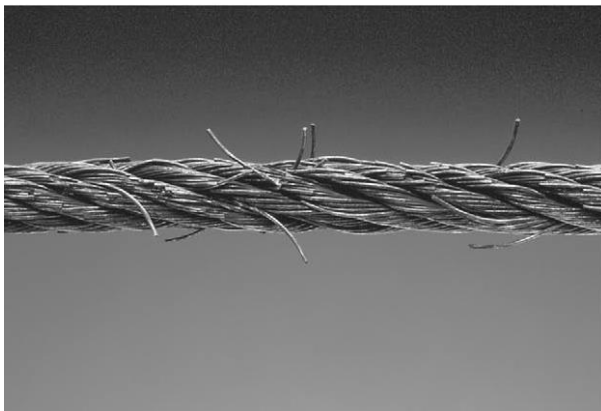
Cable With Severe Corrosion
